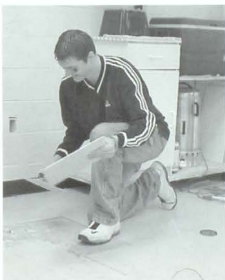
Jesse Peden putties a tile for the cafeteria floor. The buildings and trades class fixed broken tiles throughout the high school. Photo by Aaron Dunn.
